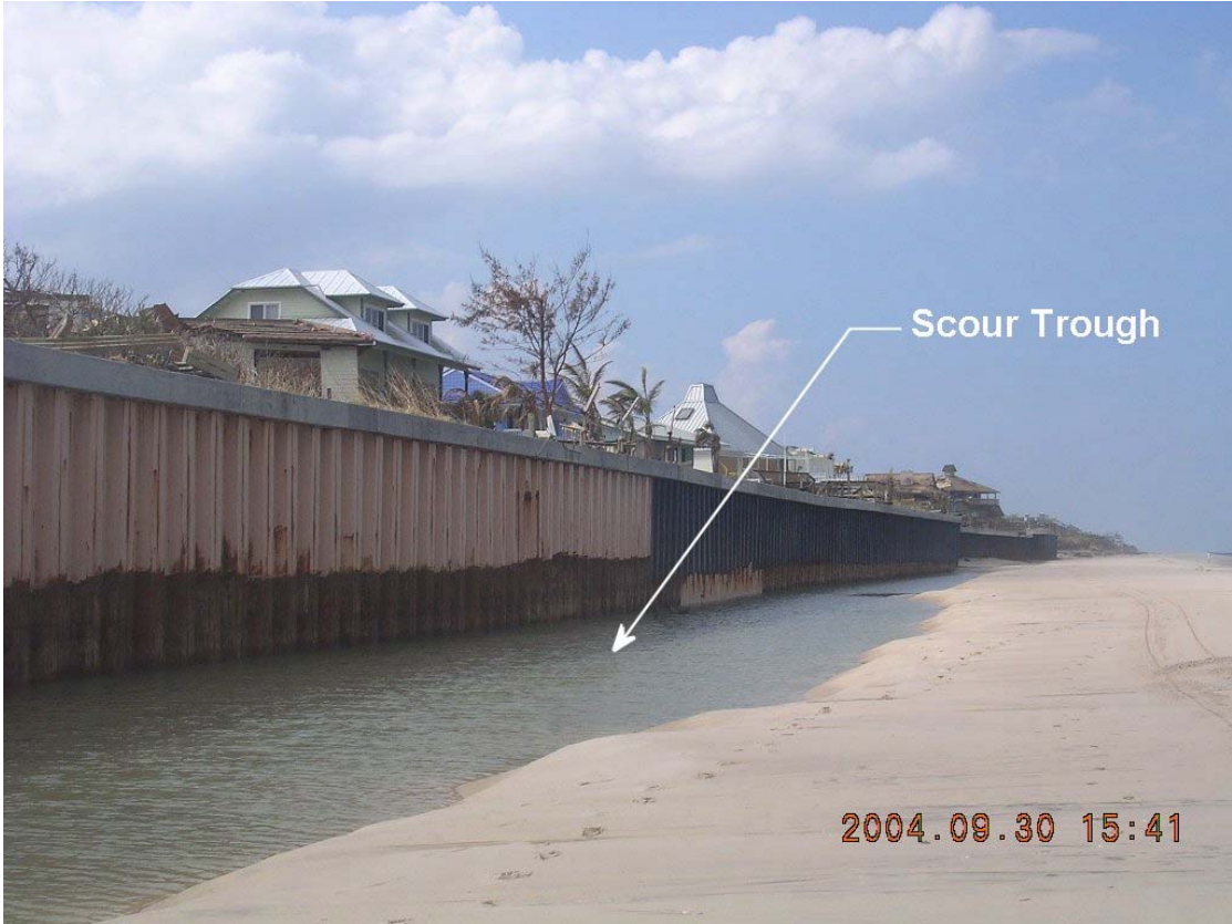
Photo 16a: Severe Beach Scour Adjacent to Summerplace Seawall
