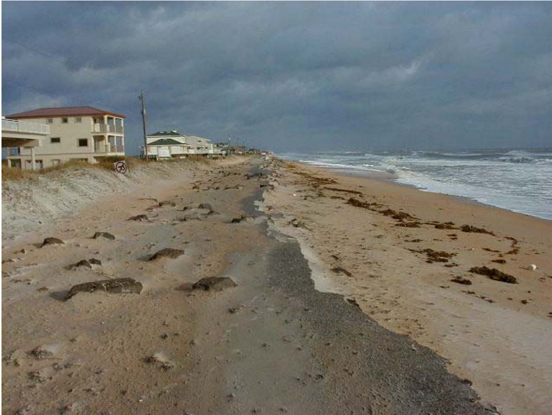
Photo 2: Summer Haven Road Damage
