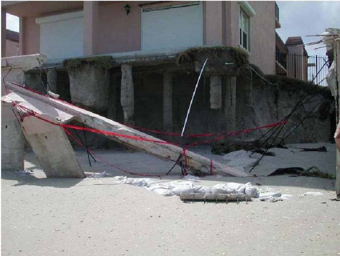
Photo 5: Building Undermined after Seawall Collapsed, New Smyrna Beach
