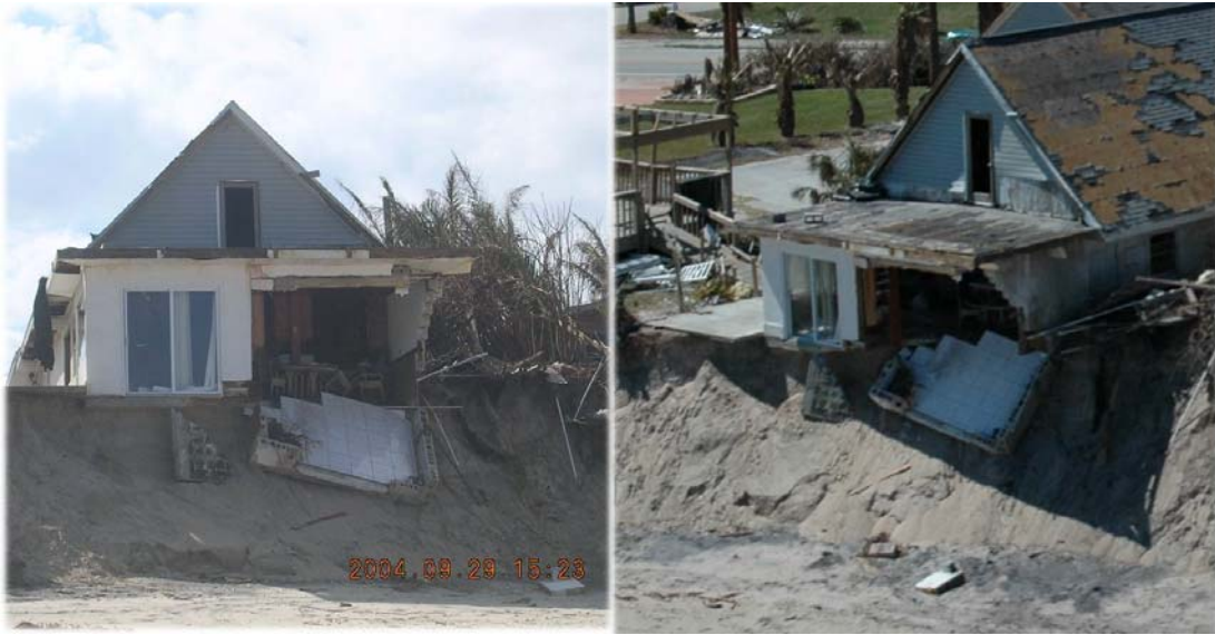
Photo 12: Slab on Grade Failure
