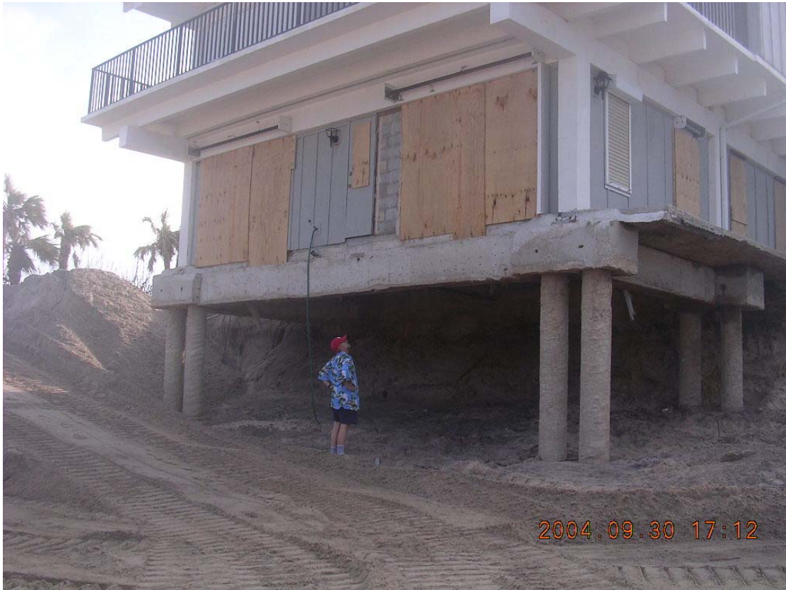
Photo 21: Undermined Condominium, Vero Beach
