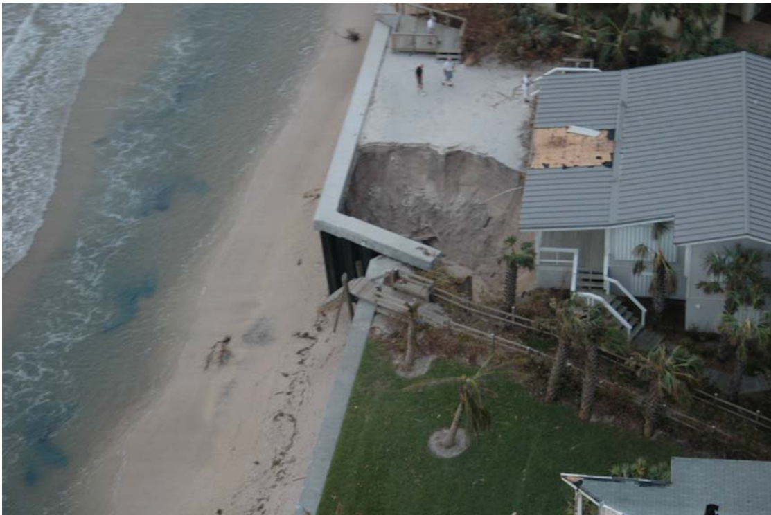
Photo 16b: Loss of Material behind Seawall
