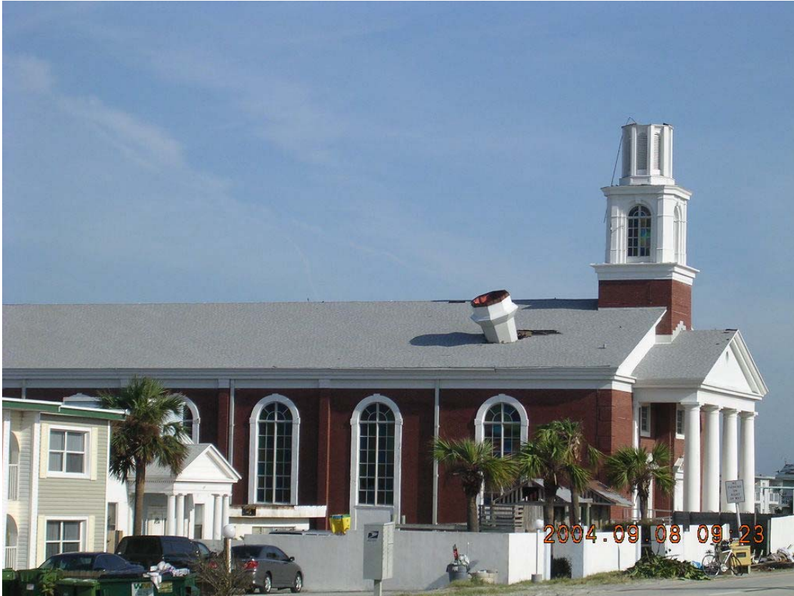
Photo 7: Roof Damage, Cocoa Beach
