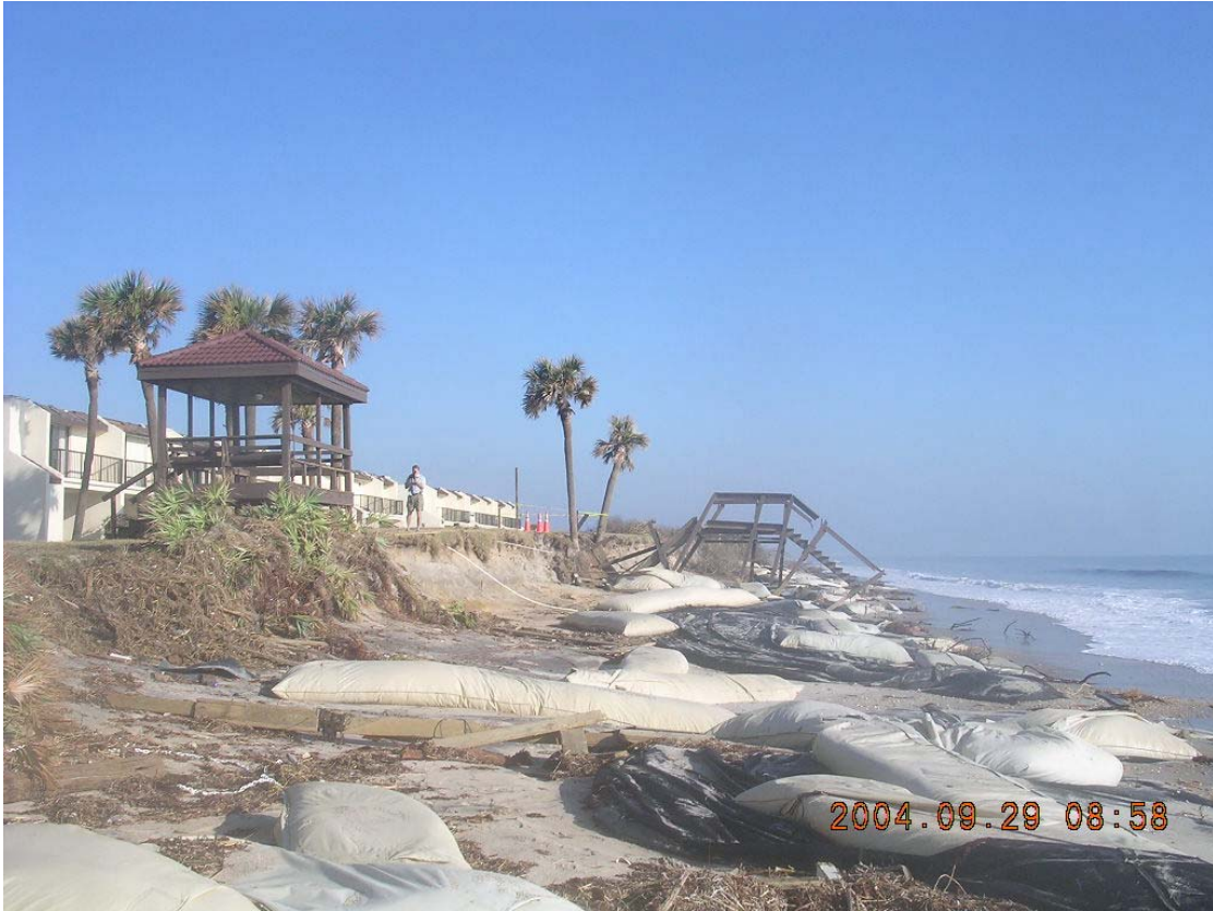
Photo 8: Pineda Causeway Condominiums Erosion and Revetment Damage
